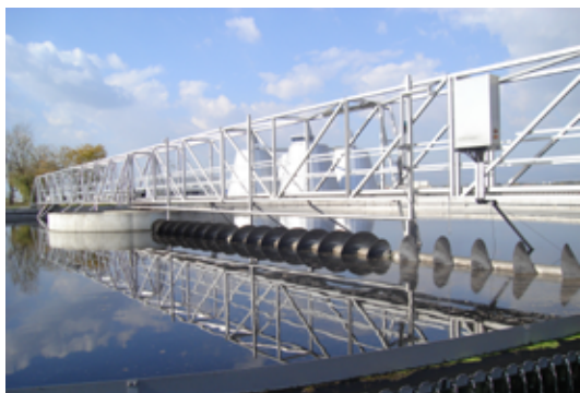
Biological wastewater treatment
